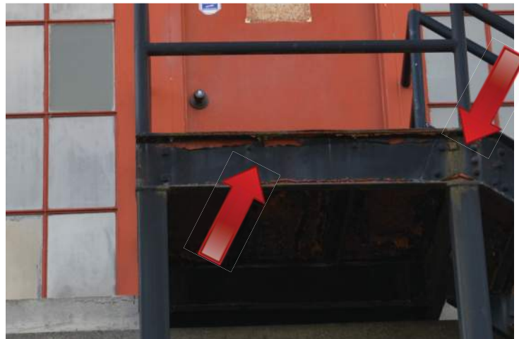
There is visible paint failure on the structure and signs of corrosion. Image by Otak. 200224 CoT CAS EL-E DSC_1039.JPG
