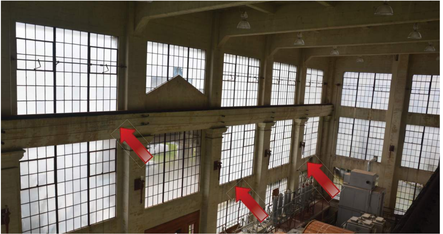
The dark areas under the windows appear to be organic growth (algae), indicating water infiltration. There is also a substantial amount of paint failure on the walls. Image by Otak. 200224 CoT CAS EL-INT DSC_0998.jpg
