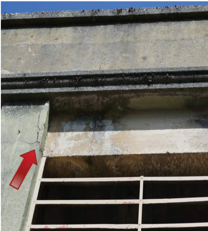
Cracking on the right edge of a pilaster on the east elevation. Image by Richaven Architecture and Preservation. 220620 CoT CAS EL-E P1000684.JPG
