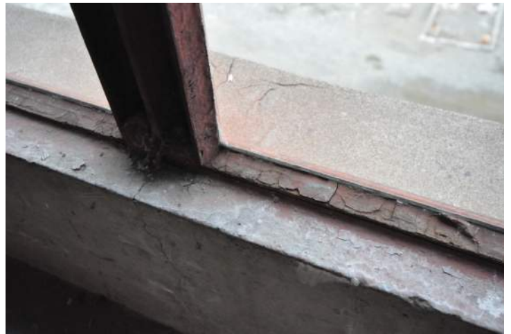
The cast-in-place steel windows exhibit extensive corrosion around the frame and loss of glazing compound. Image by Otak. 200224 CoT CAS EL-INT DSC_0092.JPG
