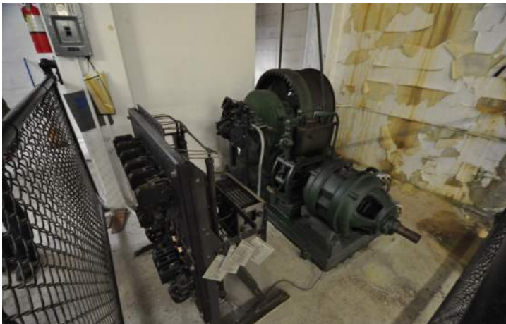
Paint failure, peeling, and soiling on walls. Image by Otak. 200224 CoT CAS EL-INT DSC_0125.JPG
