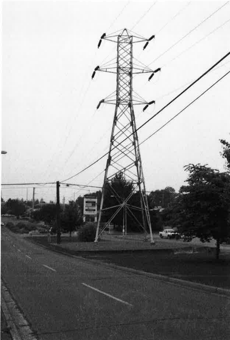
Photo 16 of 17. WA_Pierce County_Cushman Substation_0016. Typical Tower as traverses down N 21 st St.
