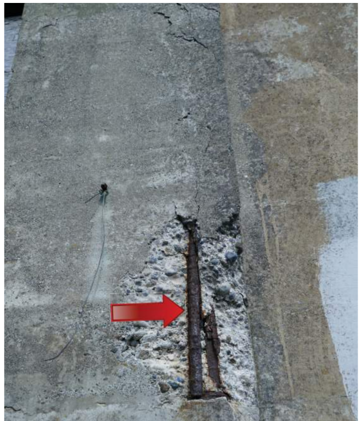
Severe separation from the substrate. Image by Richaven Architecture and Preservation. 220620 CoT CAS EL-W P1000679.JPG
