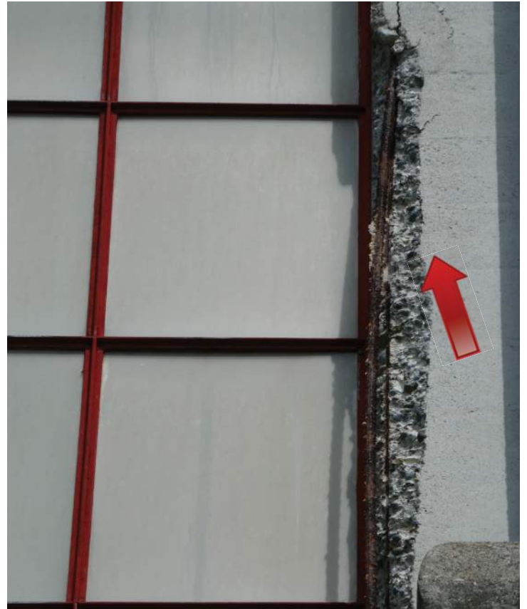
Severe spalling and separation from the substrate around a window on the west elevation. Image by Richaven Architecture and Preservation. 220620 CoT CAS EL-W P1000647.JPG
