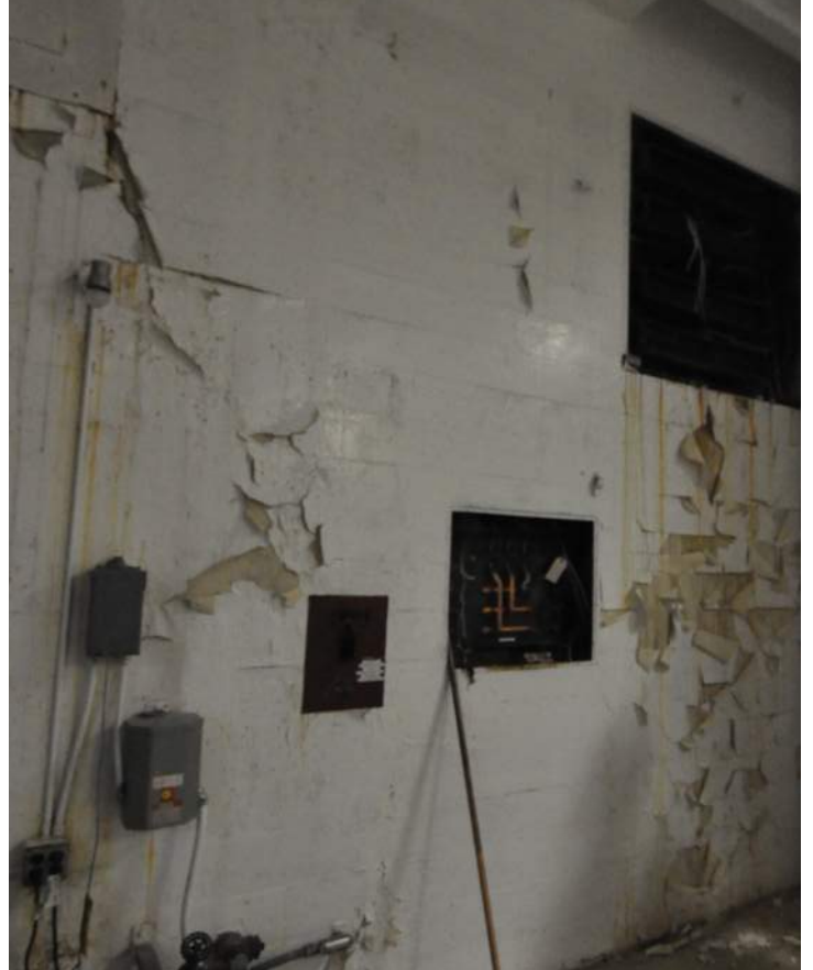
The location above shows concrete wall with the coating failing and peeling. Image by Otak. 200224 CoT CAS EL-INT DSC_0126.JPG.
