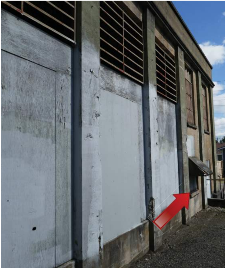
Metal louvers on the west elevation and a missing window covered with plywood boards. Image by Richaven Architecture and Preservation 06/20/22, 220620 CoT CAS EL-W P1000674.JPG
