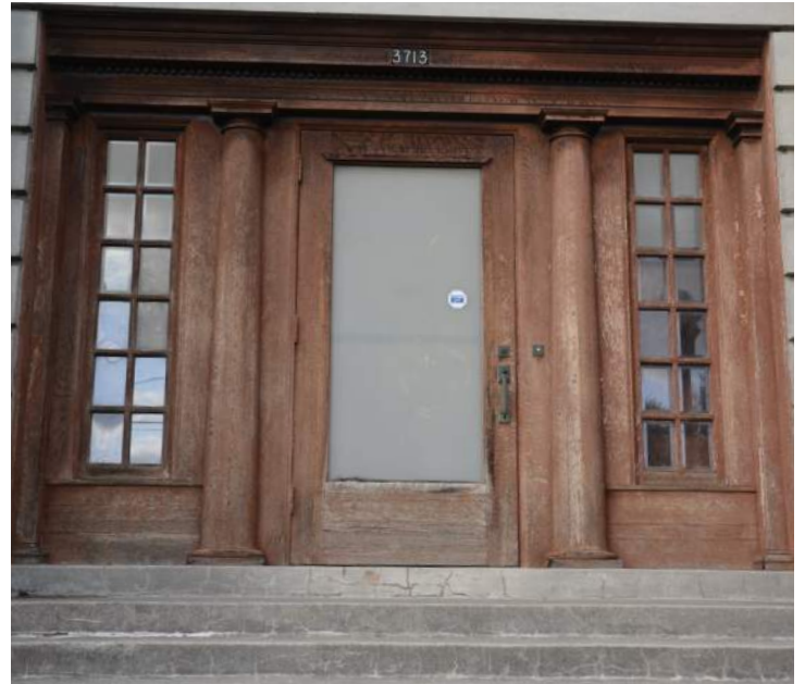
Wood columns with a significant amount of discoloration. Image by Richaven Architecture and Preservation. 200224 CoT CAS EL-S DSC_1063.JPG
