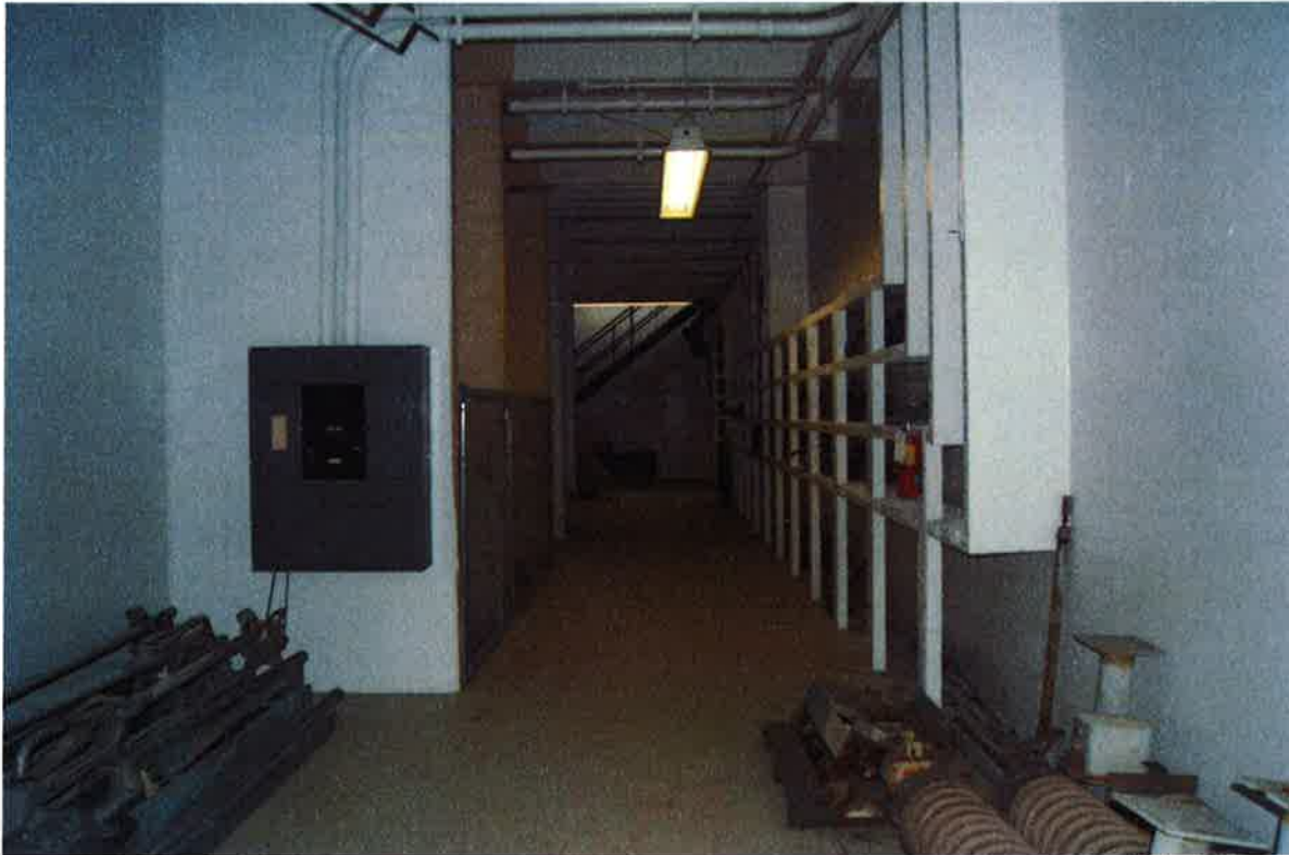
Photo 15 of 17. WA_PierceCounty_CushmanSubstation_0015. Basement level of Cushman Substation.
