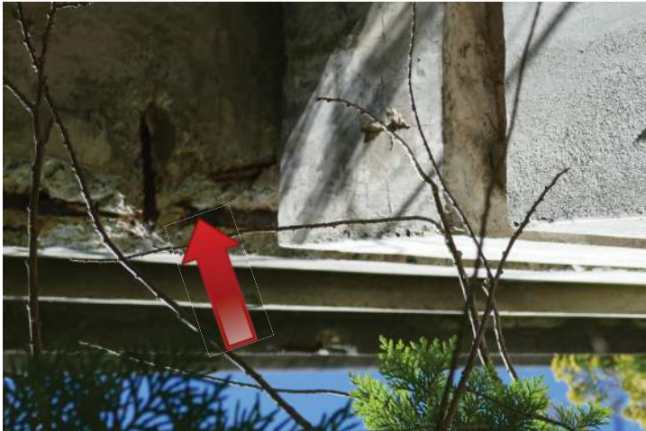
Looking up at the failed concrete at the upper left corner at a ground-level window bay, west elevation. The image below shows concrete debris that has separated from the substrate. Image by RichavenArchitectureandPreservation.220620CoTCASEL-WP1000663.JPG
