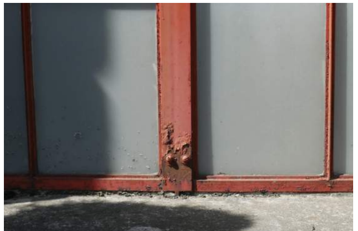
Visible corrosion around the fasteners of a window on the west elevation. Image by Richaven Architecture and Preservation. CoT CAS EL-W P1000654
