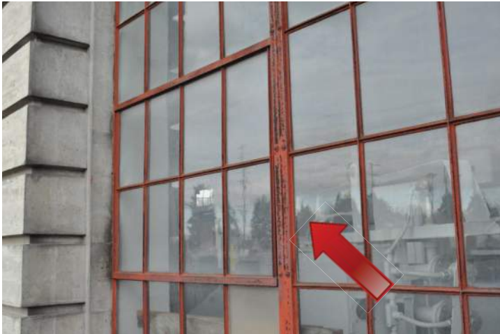
Steel with signs of corrosion. Image by Richaven Architecture and Preservation. 200224 CoT CAS EL-N DSC_0175.JPG
