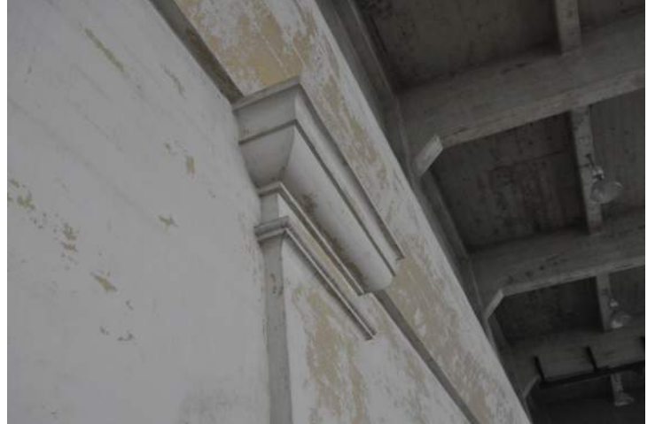
Visible paint failure, flaking, and peeling. Image by Otak. 200224 CoT CAS EL-INT DSC_0082.JPG.
