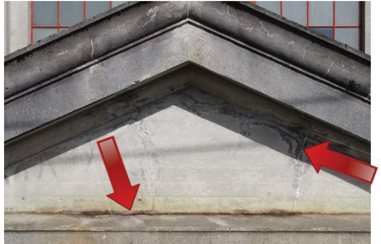
The pediment above the main entrance on the south elevation shows the build-up of atmospheric soiling that has adhered to the concrete and visible stains due to corrosion of the reinforcing steel. Efflorescence is also observed. Image by Richaven Architecture and Preservation. 200224 CoT CAS EL-S DJI_0023.JPG
