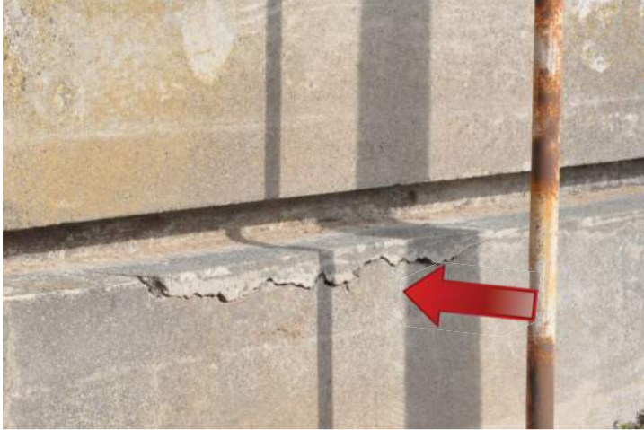
Cracks on the foundation, on the east corner of the south elevation. Image by Richaven Architecture and Preservation. 200224 CoT CAS EL-S DSC_0004.JPG
