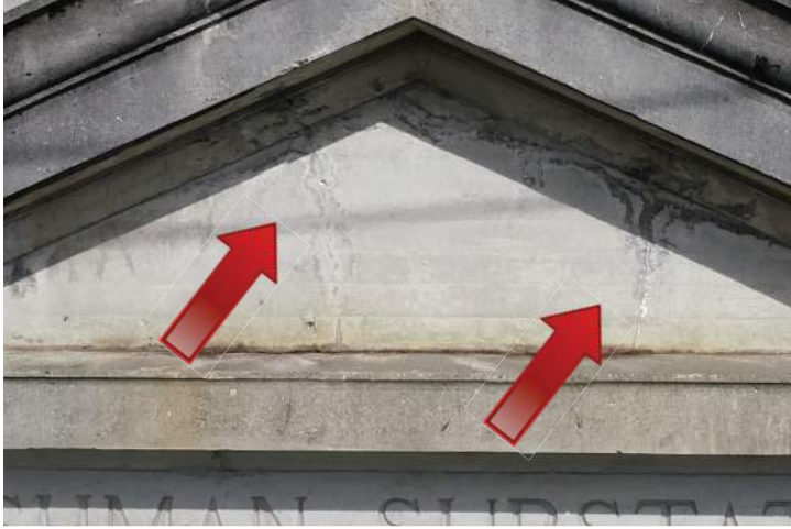
Spalling and efflorescence on the frieze. Image by Richaven Architecture and Preservation. 200224 CoT CAS EL-S DJI_00221.PNG
