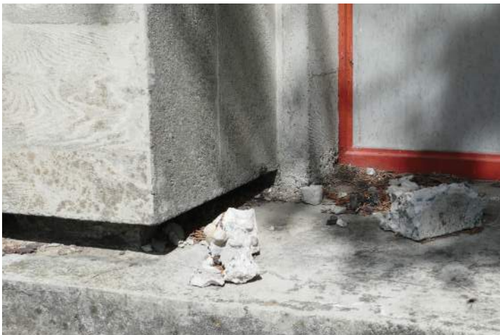
Failed concrete at one of the ground level window bays on the west elevation. Image by Richaven Architecture and Preservation. 220620 CoT CAS EL-W P1000660.JPG
