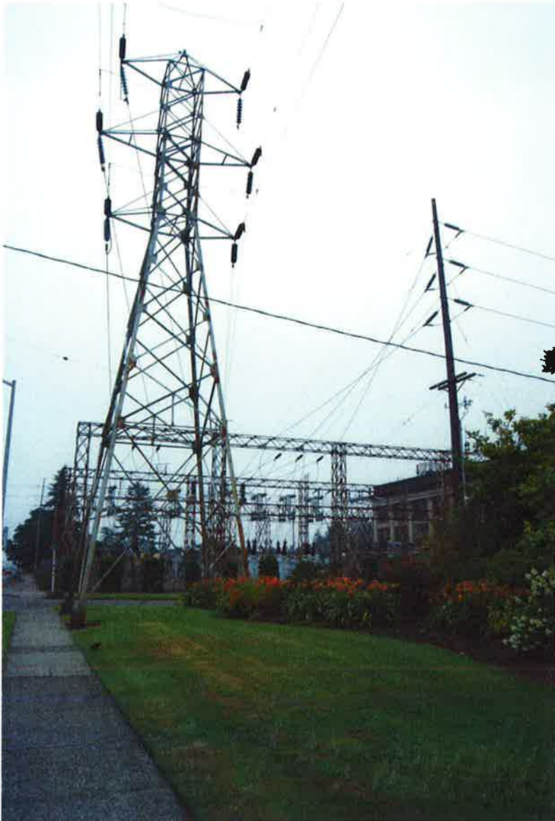
Photo 16 of 17. WA_Pierce County_Cushman Substation_0016. First Tower as it leaves/enters substation
