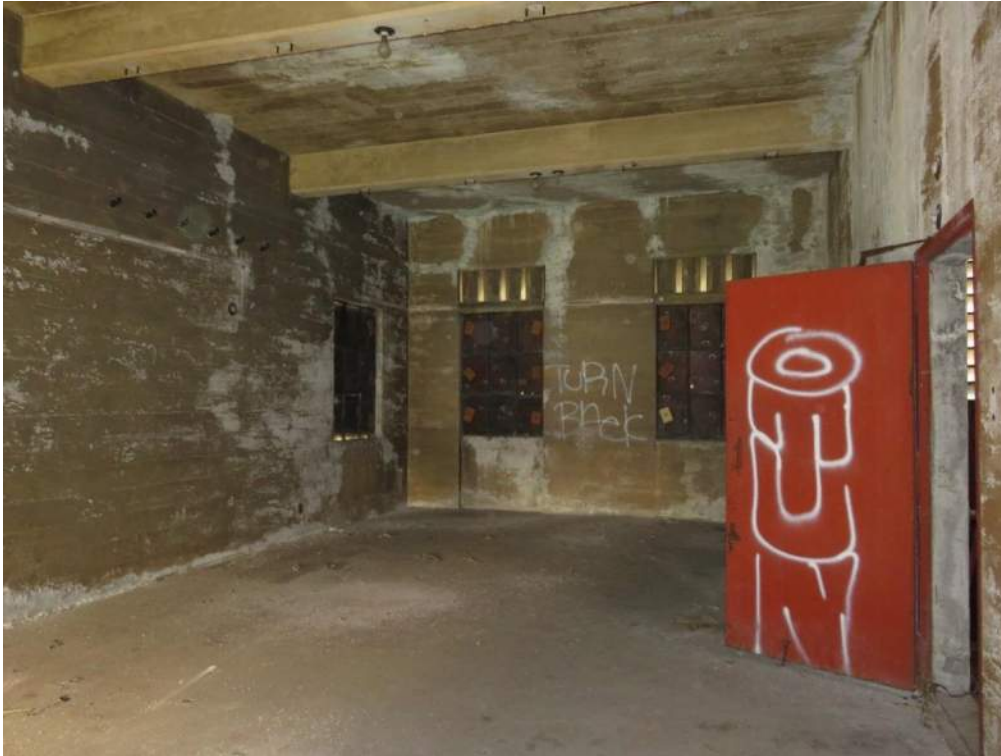
Photo 10 of 13. WA_PierceCounty_AdamsSt.Substation_0010. Adams St. Substation, interior, switch room, upper level, view west.
