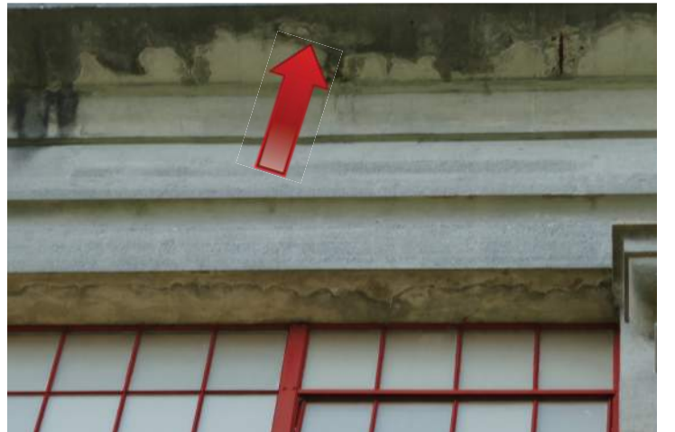
Build-up of airborne pollutants that have adhered and stained the concrete under the cornice on the south elevation. Efflorescence is also observed. Image by Richaven Architecture and Preservation. 220620 CoT CAS EL-W P1000666.JPG
