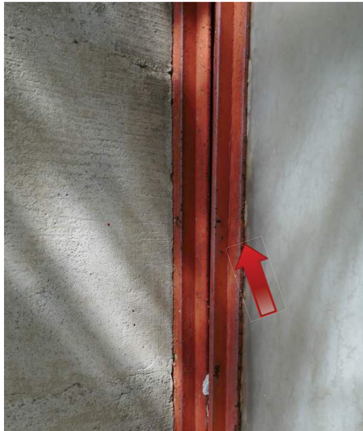
Detail of the cast-in-place steel window frame exhibits delamination, corrosion, and missing glazing compound. Image by Richaven Architecture and Preservation. 220620 CoT CAS EL-W P1000664.JPG
