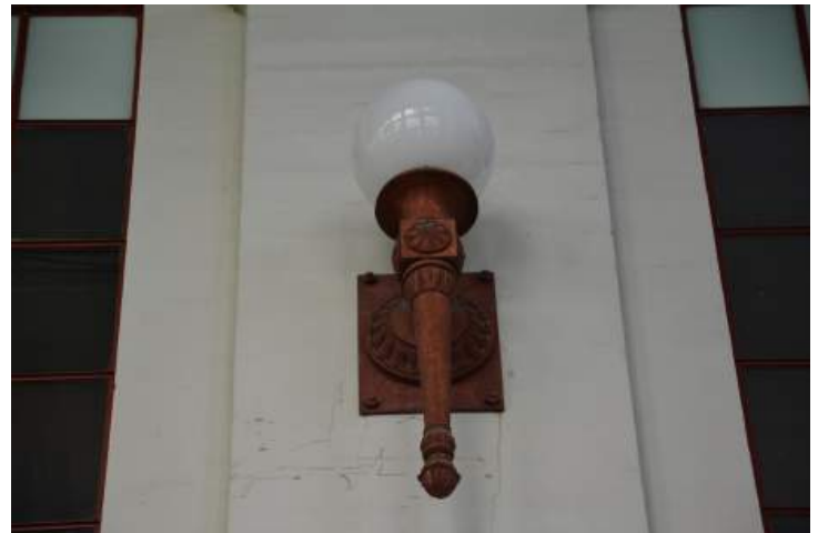
Cast iron decorative light fixture exhibiting corrosion. Image by Otak. 200224 CoT CAS INT DSC_0970.JPG
