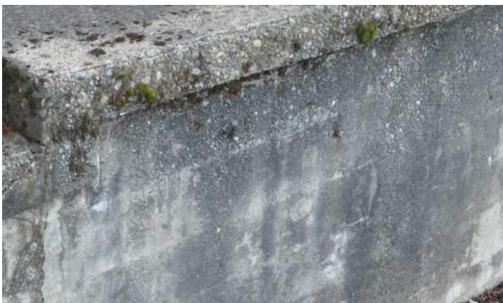
Organic soiling (algae and plants) and atmospheric soiling were observed on concrete at the West elevation of the building. Image by Richaven Architecture and Preservation. 200224 CoT CAS EL-W DSC_0047.JPG
