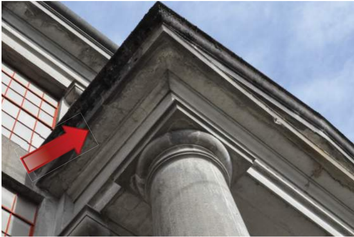
Efflorescence was observed under the pediment and entablature on the main entrance. Image by Richaven Architecture and Preservation. 200224 CoT CAS EL-S DSC_0016.JPG
