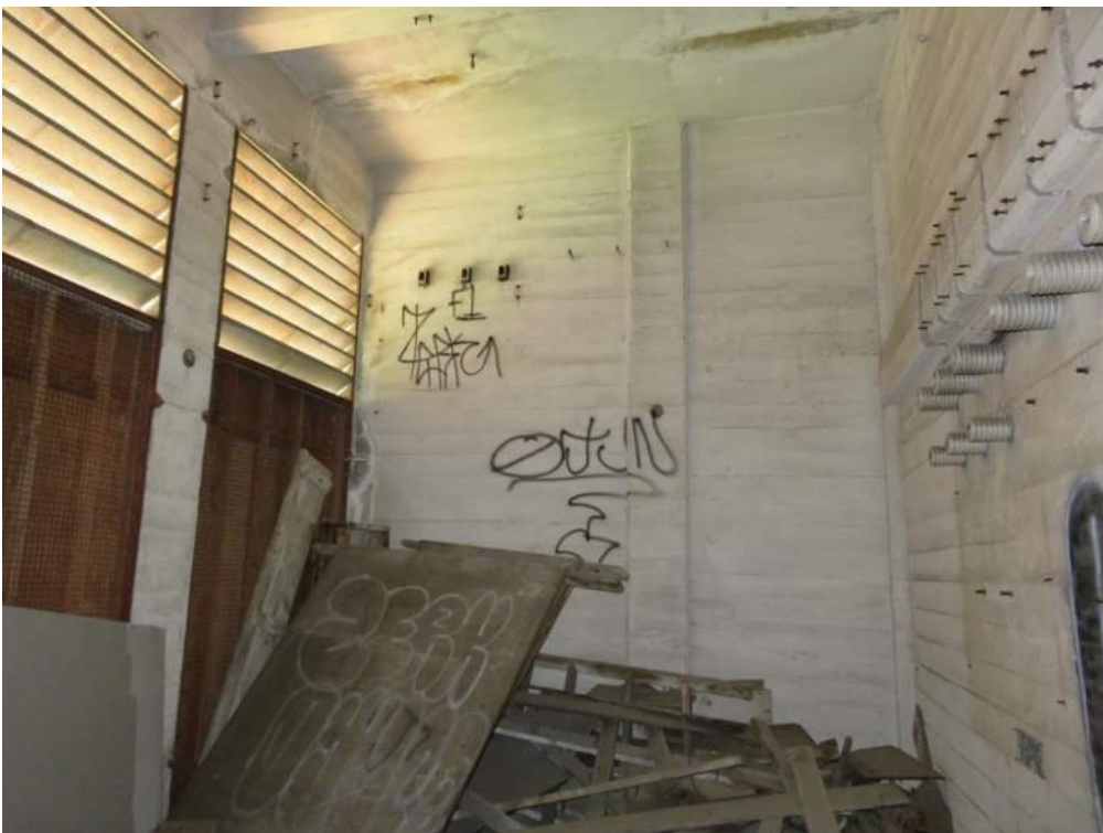
Photo 13 of 13. WA_PierceCounty_AdamsSt.Substation_0013. Adams St. Substation, interior, transformer room, view north.
