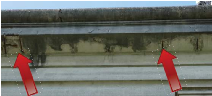
Exposed reinforcing steel and spalling under the cornice on the west elevation. Image by Richaven Architecture and Preservation. 220620 CoT CAS EL-W P1000666.JPG
