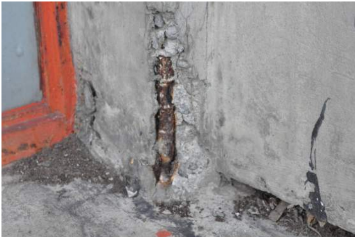
Exposed reinforcing steel with corrosion. Image by Richaven Architecture and Preservation. 200224 CoT CAS EL-N DSC_0174.JPG
