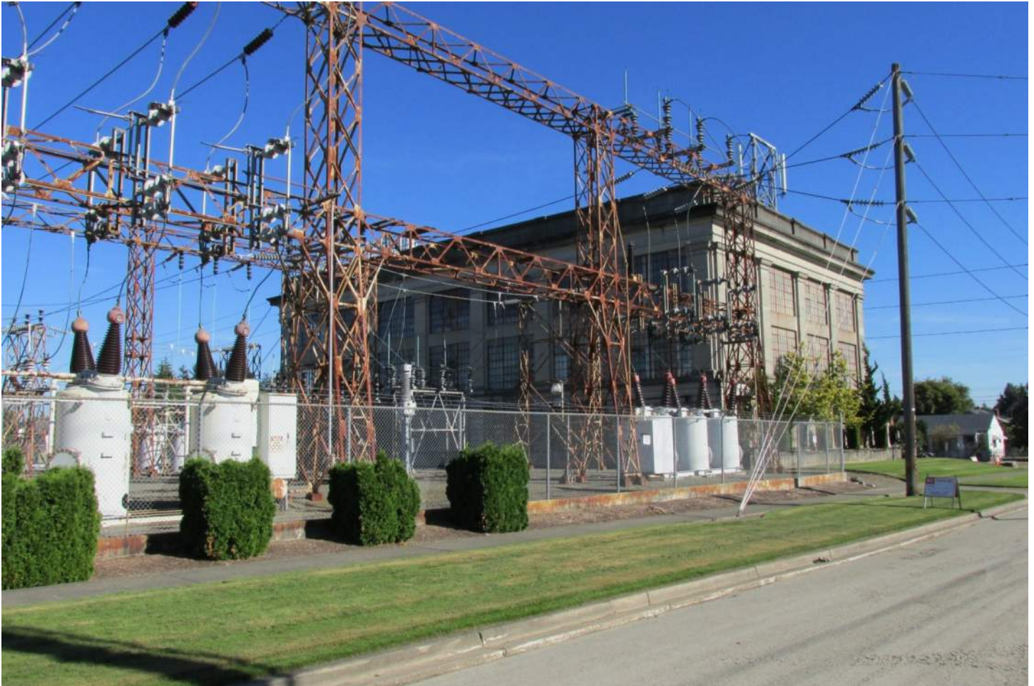
Figure 19 Cushman Substation view southeast
