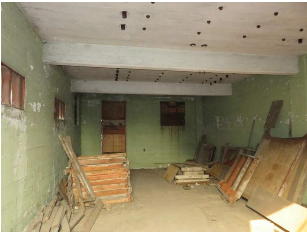
Photo 9 of 13. WA_PierceCounty_AdamsSt.Substation_0009. Adams St. Substation, interior, regulator room, lower level, view west.
