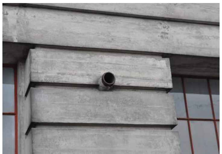
The tube embedded in the concrete appears not to be adequately sealed. It will allow water infiltration into the wall. 200224 CoT CAS EL-N DSC_0183.JPG
