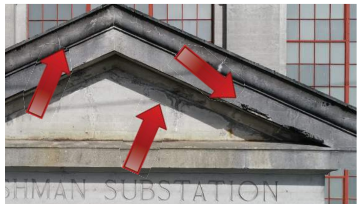
Pediment above the main entrance on the south elevation shows severe spalling, efflorescence, and atmospheric soiling. Image by Richaven Architecture and Preservation. 200224 CoT CAS EL-S DJI_00221.PNG
