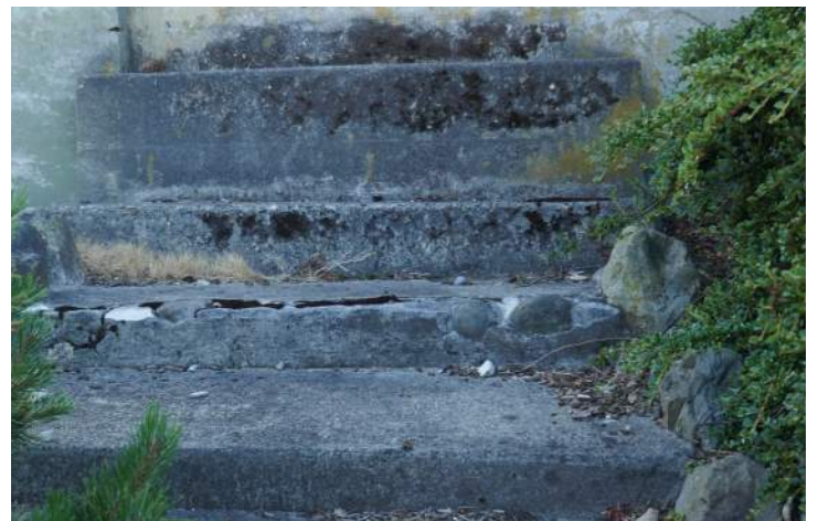
Organic soiling (algae and plants), observed on concrete stairs on the east elevation of the building. Image by Richaven Architecture and Preservation. 220620 CoT CAS EL-E P1000689.JPG
