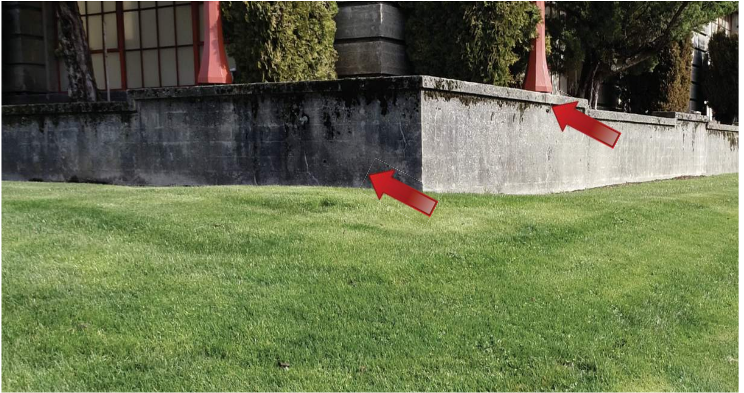
A substantial amount of organic soiling (algae) and atmospheric soiling was observed on walls on the west and south elevations. Image by Richaven Architecture and Preservation. 200224 CoT CAS EL-S-W 200224 CoT CAS EL-S-W DJI_0028.PNG
