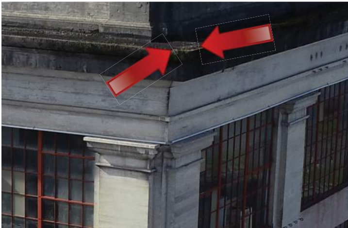
Water proofing on top of cornice, on the east corner of the south elevation appears to be failing. Image by Richaven Architecture and Preservation. 200224 CoT CAS EL-S-W DJI_00036.jpg
