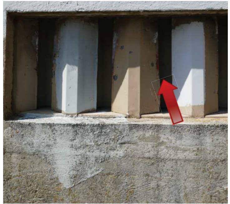
Vent on the south elevation with corrosion on the edges. Areas in white were painted to cover graffiti. Image by Richaven Architecture and Preservation. P000673.JPG.
