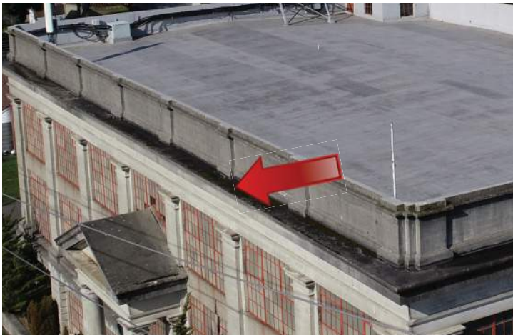
Algae growth on the cornice on the south elevation indicates that water is collecting. Image by Richaven Architecture and Preservation. 200224 CoT CAS EL-S DJI_0037.JPG
