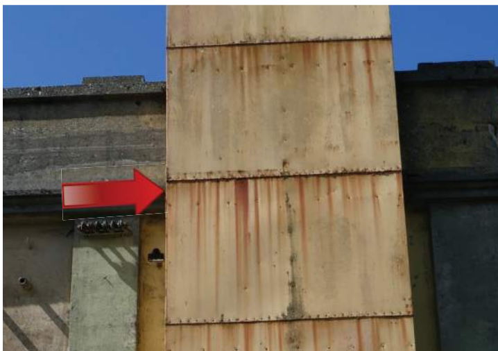
The panels that form the steel ventilation stack are severely corroded. Image by Richaven Architecture and Preservation. 220620 CoT CAS EL-S P1000671.JPG
