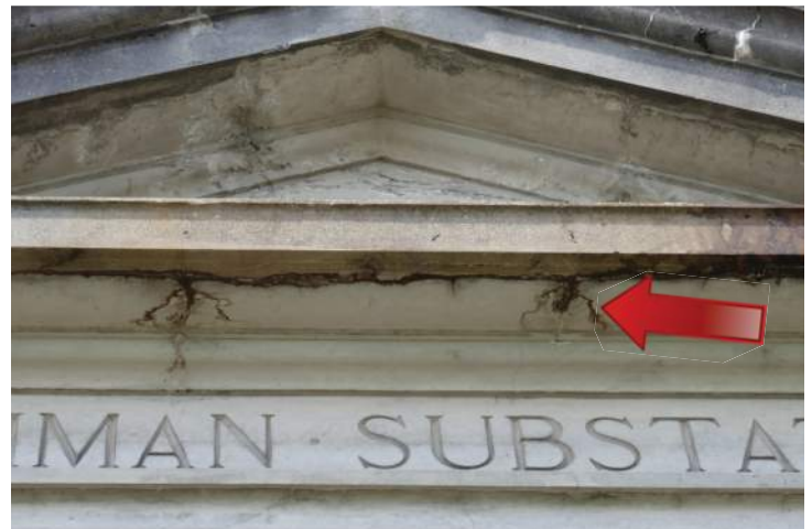
The pediment above the main entrance on the south elevation shows some water damage that resulted in cracking and spalling of the concrete. Image by Richaven Architecture and Preservation. 220620 CoT CAS EL-S P1000651.JPG
