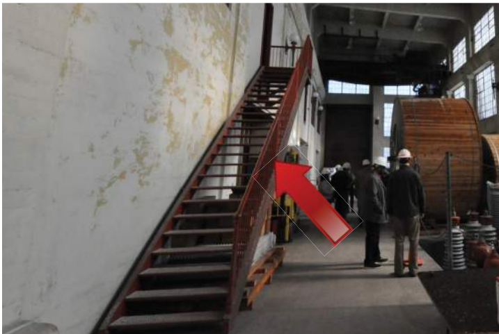
Dust / dirt soiling was observed on the stairwell. Image by Otak. 200224 CoT CAS EL-INT DSC_0065.JPG
