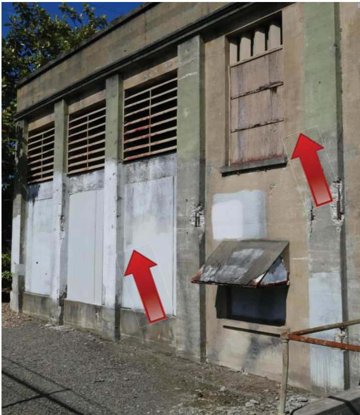
Missing windows and openings for ventilation under the louvers have been covered with plywood boards. Historical photos show single steel-framed nine-light windows with louvered vents above. Image by Richaven Architecture and Preservation. 220620 CoT CAS EL-W P1000685.JPG
