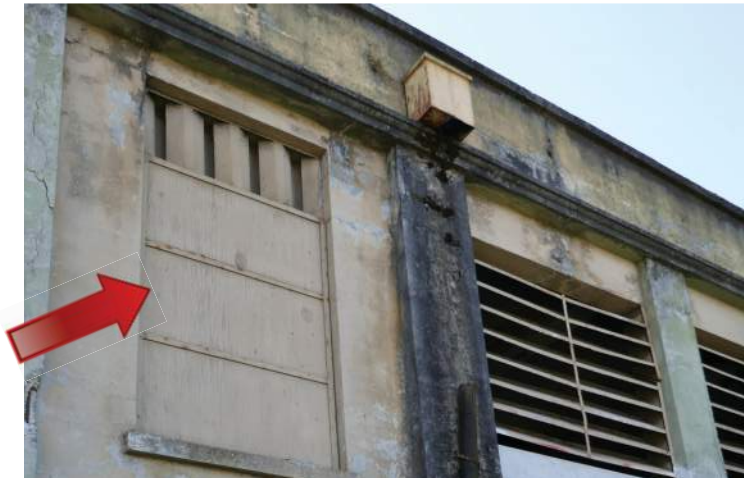
Missing steel windows and vents have been covered with plywood boards. Image by Richaven Architecture and Preservation. 220620 CoT CAS EL-E P1000691.JPG.
