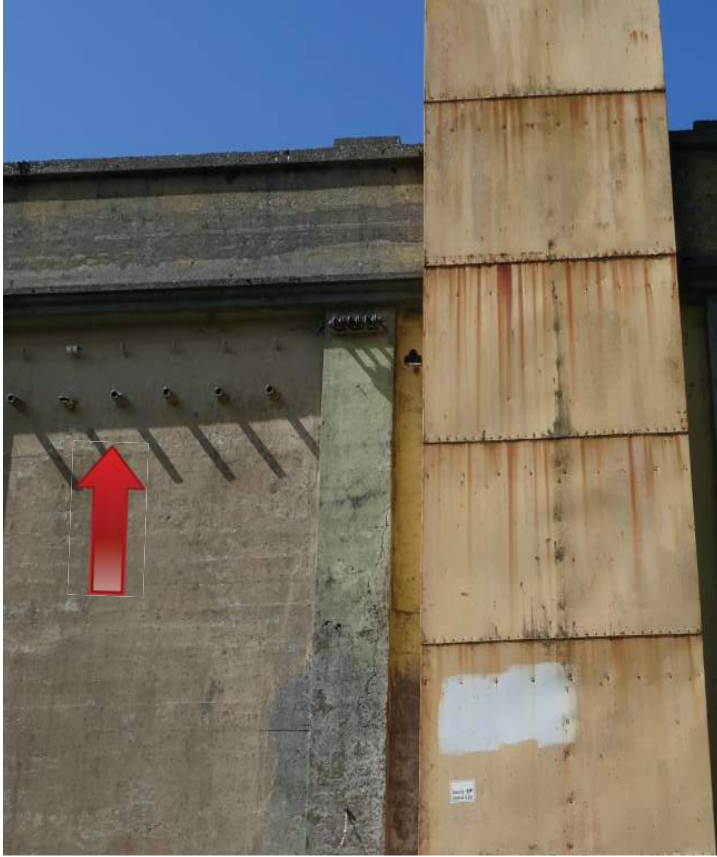
Observed steel eye bolts, pulleys, and severed tubes embedded into the concrete on the south elevation. The pipes embedded in the concrete appear not to be adequately sealed, allowing water infiltration into the wall. Image by Richaven Architecture and Preservation. 220620 CoT CAS EL-S P1000671.JPG
