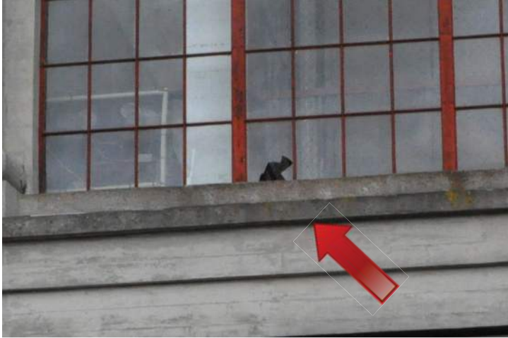
Broken glass pane on window bay above rolling gate on the north elevation. Image by Richaven Architecture and Preservation 200224 CoT CAS EL-N DSC_0189.JPG
