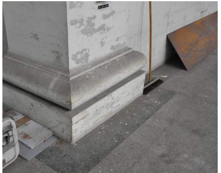
Paint failure and dust / dirt soiling on the base of the pilaster. Image by Otak. 200224 CoT CAS EL-INT DSC_0078.JPG
