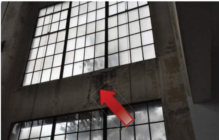
Soiling under the window appears to be mold and signs of water infiltration. Image by Otak. 200224 CoT CAS EL-INT DSC_0070.JPG
