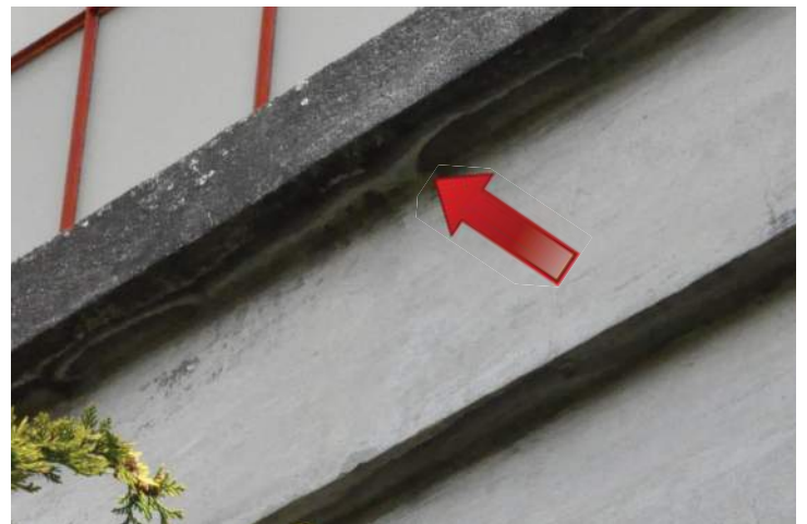
Efflorescence under a window ledge on the west elevation. Moisture infiltration will result in spalling. Image by Richaven Architecture and Preservation. 200224 CoT CAS EL-W DSC_0034
