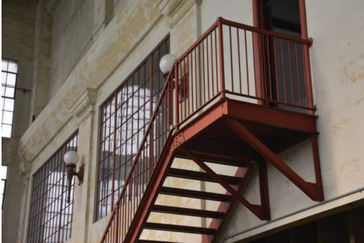
The stairwell railings are in fair condition. No corrosion was observed. Image by Otak. 200224 CoT CAS INT DSC_0977.JPG
