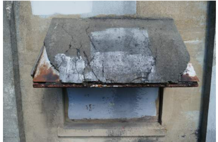
The metal awning on the west elevation is corroded. A layer of asphaltic material attached to its surface is severely damaged. Image by Richaven Architecture and Preservation. 220620 CoT CAS EL-W P1000680.JPG
