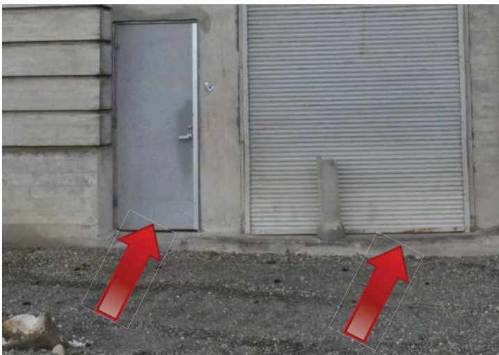
Doors on the north elevation are beginning to deteriorate. Image by Richaven Architecture and Preservation. 200224 CoT CAS EL-S DSC_0189.JPG
