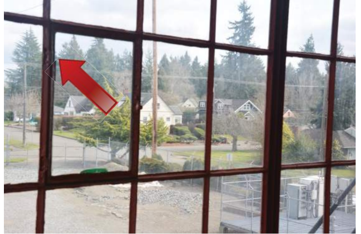
Badly corroded steel window frames and loss of glazing compound. Image by Otak. 200224 CoT CAS EL-INT DSC_10099.jpg
