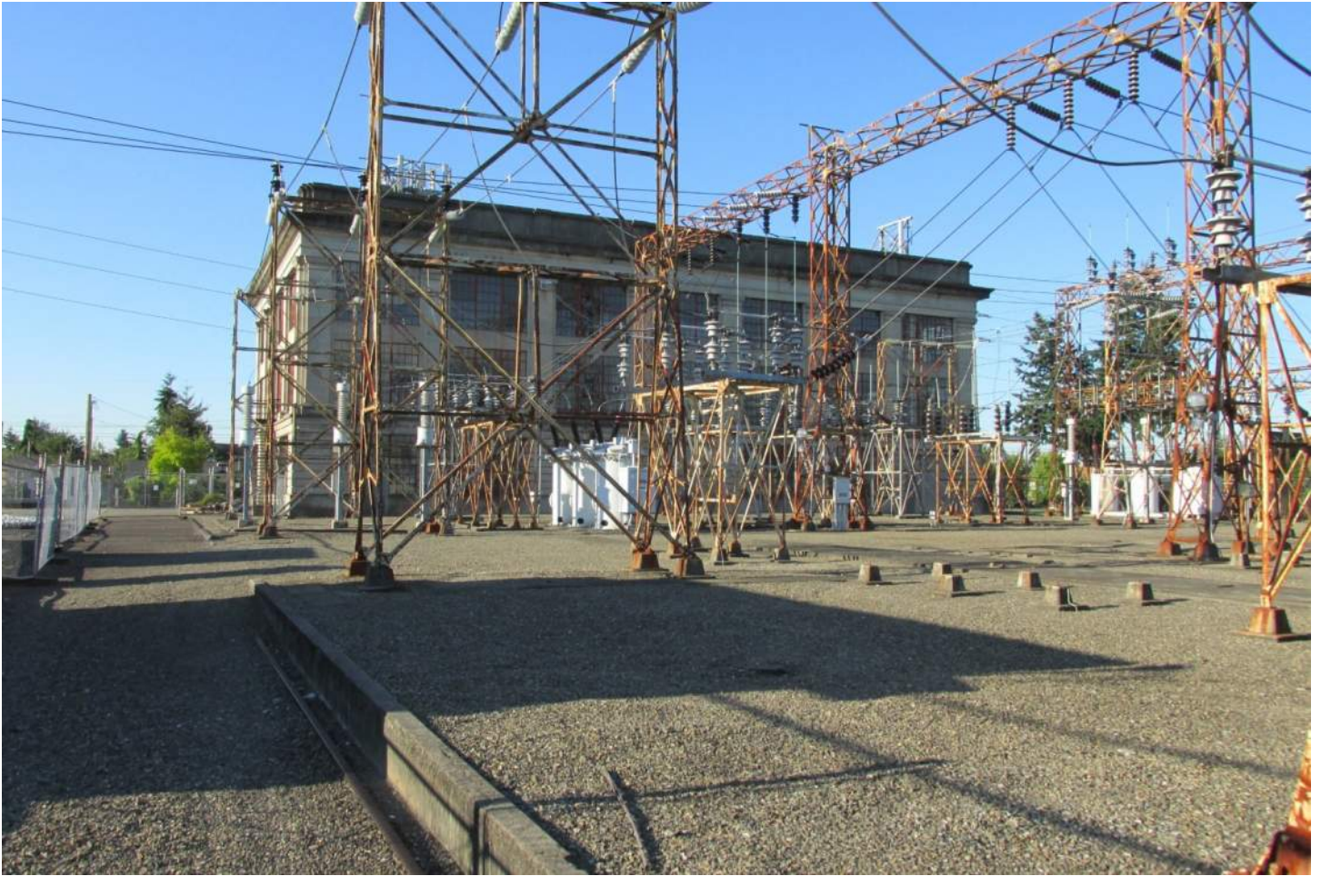
Figure 20 Cushman Substation view south
