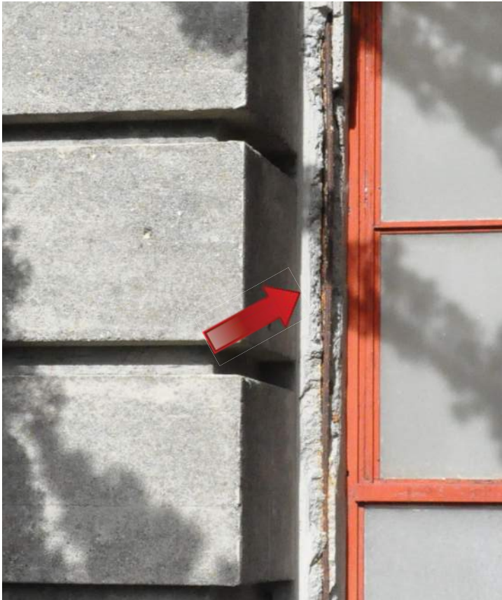
Spalling around a window frame on the west elevation and reinforcing steel bar exposed due to carbonation-induced corrosion. Often occurs in areas with a shallow concrete cover Image by Richaven Architecture and Preservation. 200224 CoT CAS EL-W DSC_0026.JPG
