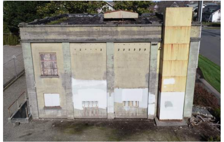
View of south elevation. White paint has been applied to the concrete walls to cover graffiti. Image by Richaven Architecture and Preservation. 200224 CoT CAS EL-S DJI_0071.JPG
