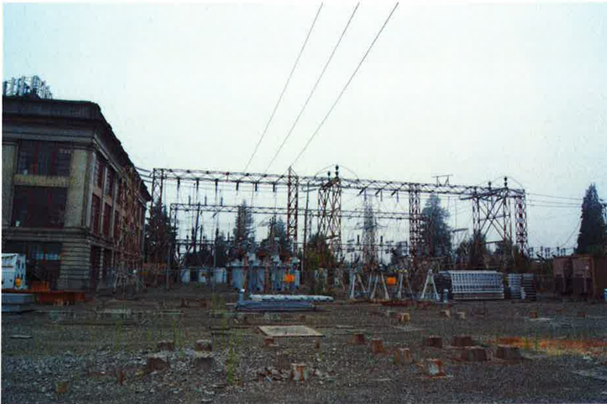
Photo 6 of 17. WA_PierceCounty_CushmanSubstation_0006. Viewing west to the exterior, modern switchyard (noncontributing) at Cushman Substation.
