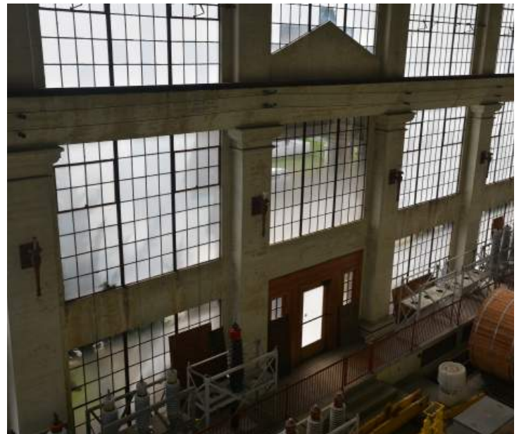
Glass globes are missing on the light fixtures above the main entrance. Image by Otak. 200224 CoT CAS EL-INT DSC_0999.JPG
