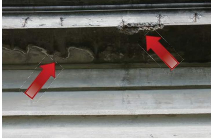
Section of the cornice on the west elevation shows spalling and reinforcing steel exposed due to water infiltration. Image by Richaven Architecture and Preservation. 220620 CoT CAS EL-W P1000649.JPG
