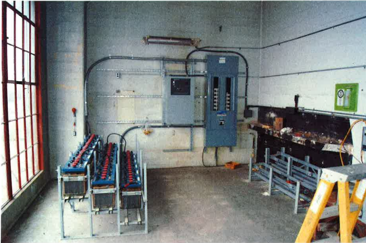
Photo 13 of 17. WA_PierceCounty_CushmanSubstation_0013. Battery room at Cushman Substation.
