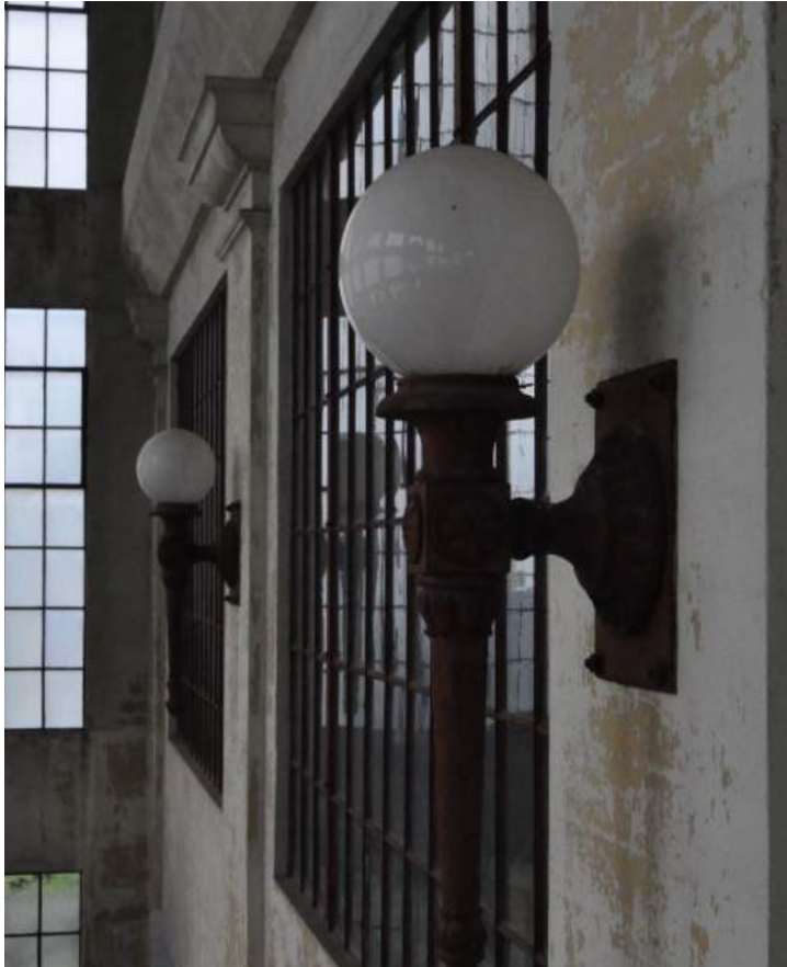
Visible paint failure in large areas in interior walls. Image by Otak. 200224 CoT CAS EL-INT DSC_0083.JPG
