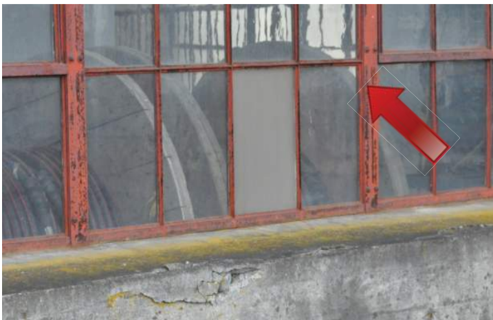
Mullions and muntins on all elevations exhibit corrosion and coating failure. Image by Otak. 200224 CoT CAS EL-N DSC_0184.JPG
