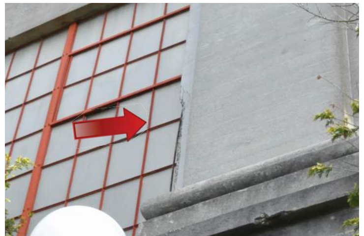
Severe separation from the substrate on the left edge of a pilaster on the west elevation. Image by Richaven Architecture and Preservation. 200224 CoT CAS EL-W DSC_0036.JPG
