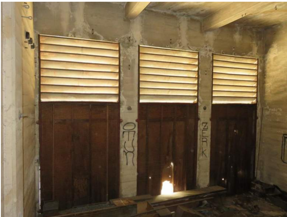
Photo 11 of 13. WA_PierceCounty_AdamsSt.Substation_0011. Adams St. Substation, interior, transformer room, view west.
