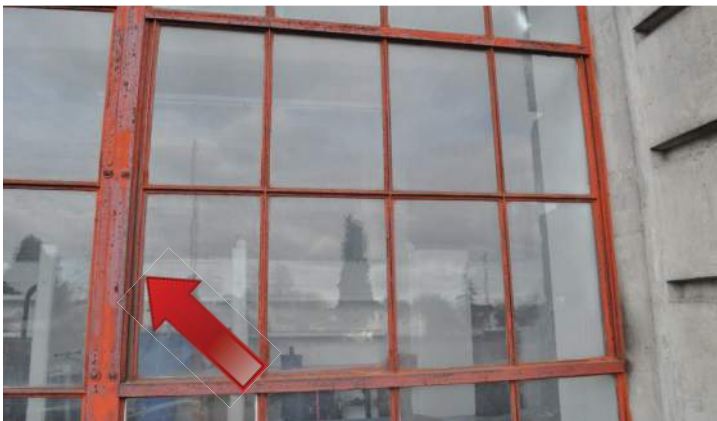
Operable sash-center-pivot exhibits corrosion and coating failure. Image by Richaven Architecture and Preservation. 200224 CoT CAS EL-N DSC_0176.JPG
