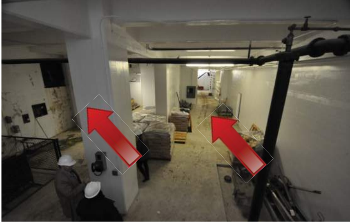
Paint failure on walls and soiling on the floor in the basement. Image by Otak. 200224 CoT CAS EL-INT DSC_0124.JPG
