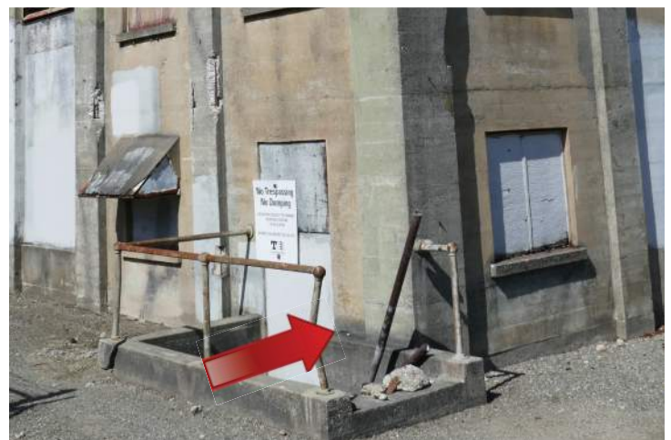
Pipe railings around the concrete stairway on the west elevation have failed. Image by Richaven Architecture and Preservation. 220620 CoT CAS EL-S-W P1000688.JPG
