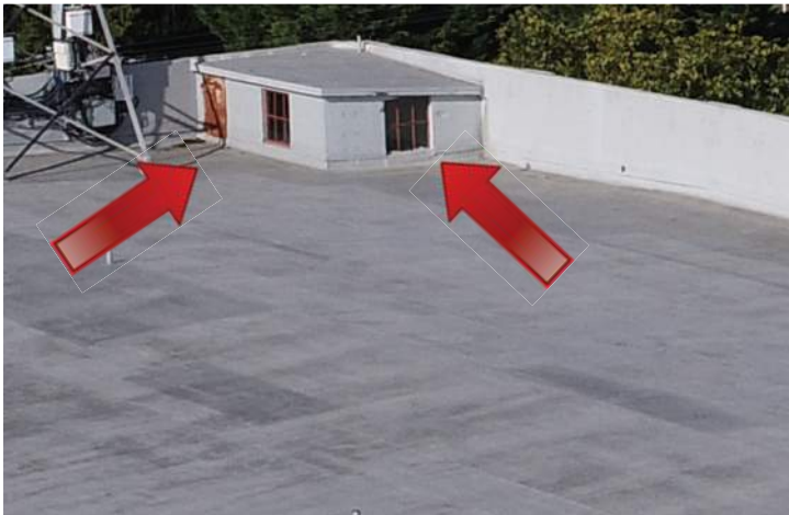
The door for roof access is badly corroded, and windows are starting to deteriorate. 200224 CoT CAS EL-S DJI_0037
