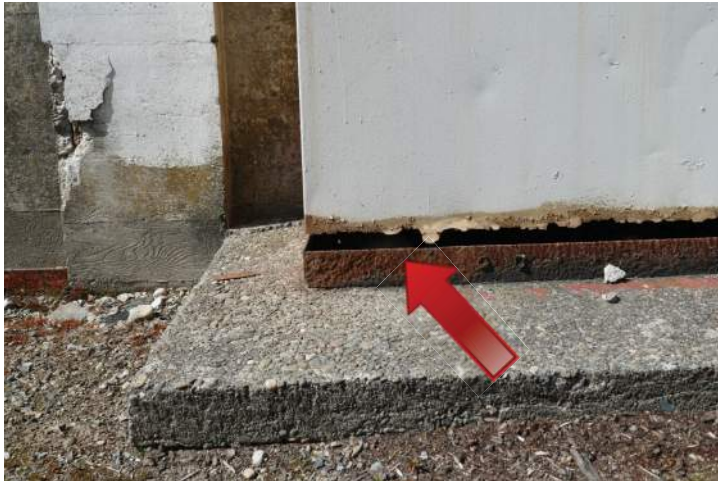
Richaven observed severe corrosion on the base of the steel ventilation stack on the south elevation. Image by Richaven Architecture and Preservation. 220620 CoT CAS EL-S P1000670.JPG
