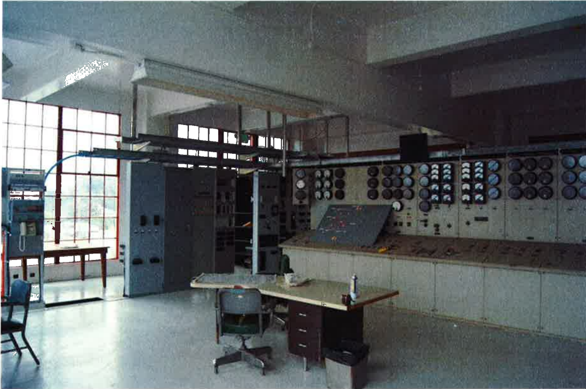
Photo 11 of 17. WA_PierceCounty_CushmanSubstation_0011. Former control room at Cushman Substation. The equipment is modern, though the room retains its original function.
