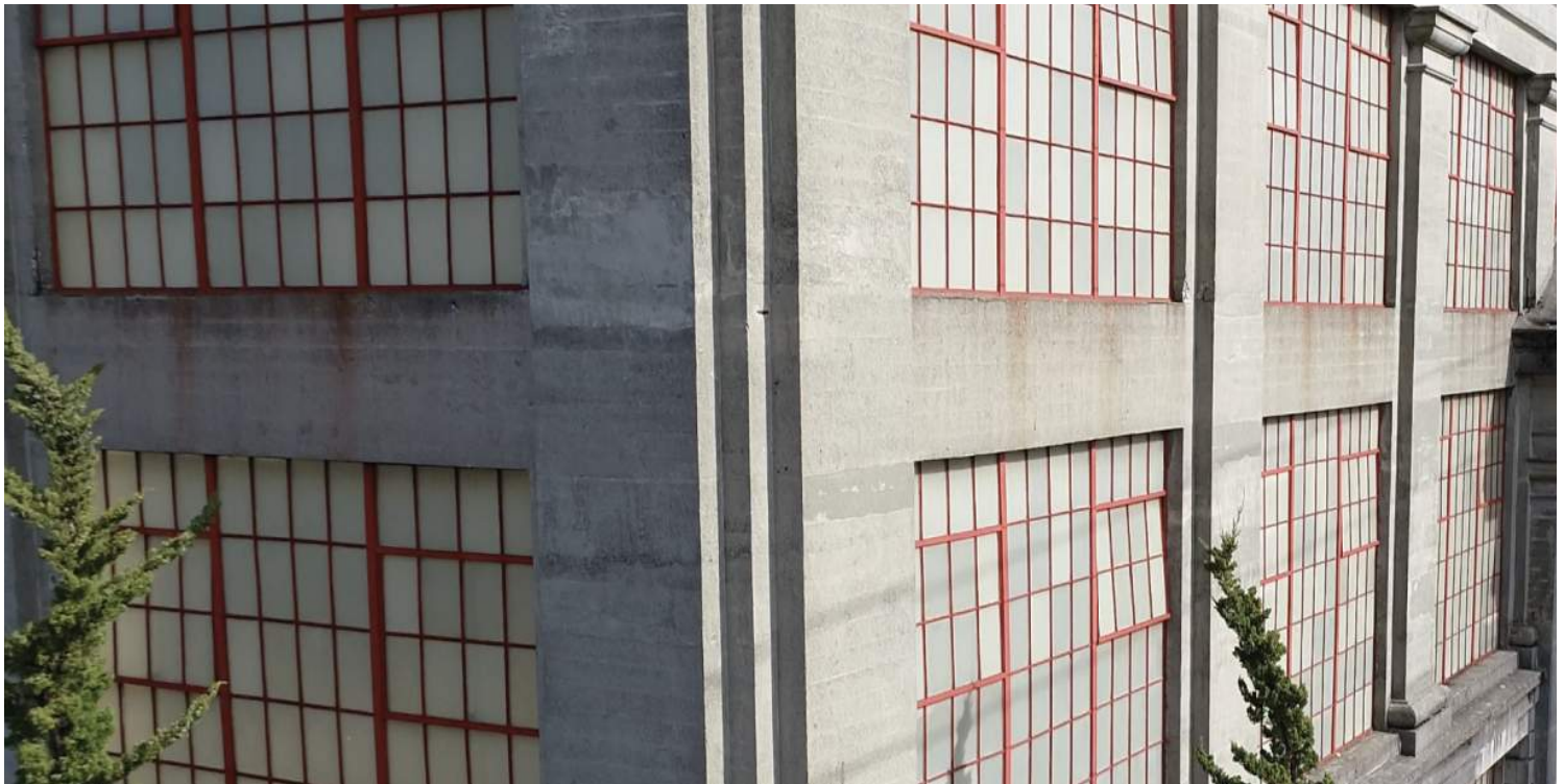
Bleeding marks of rust and paint have stained the concrete surfaces on all elevations of the building. 200224 CoT CAS EL-S-W 200224 CoT CAS EL-S-W DJI_00281.PNG
