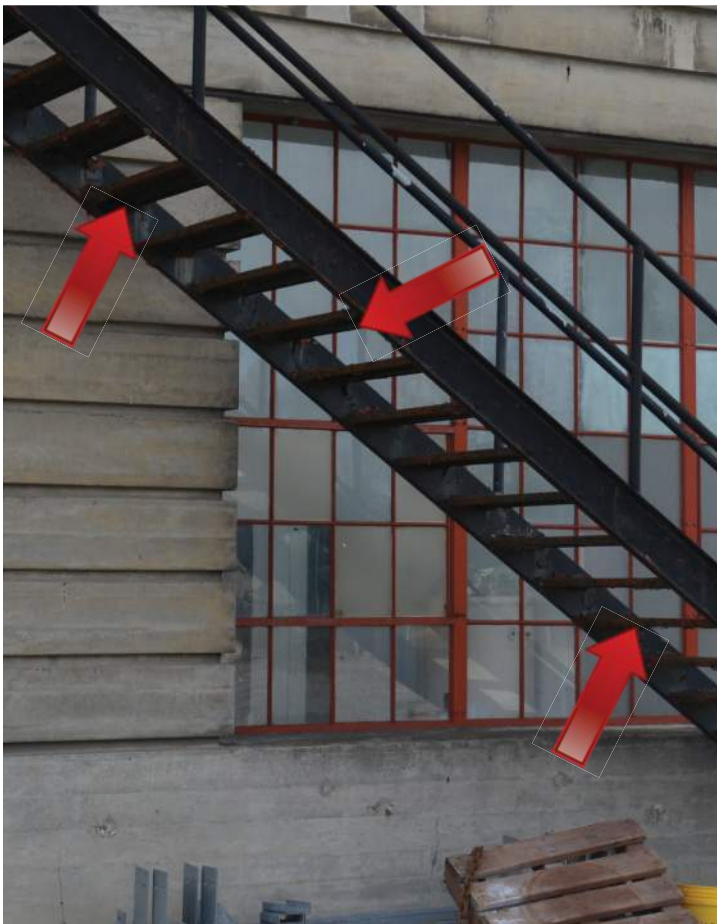
Richaven observed a substantial amount of corrosion on the steps and railings of the stairwell structure. Image by Otak. 200224 CoT CAS EL-E DSC_1045.JPG
